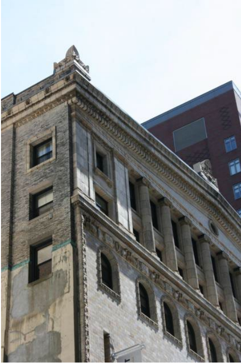
Figure 8. Northwest corner of building (north and façade elevations), 5th through 8th floors and detail of roof edge.
